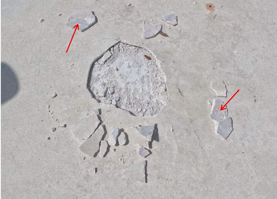
Photo No. 7 – This area looks to be both failure of plaster and bond coat together. (2026)
