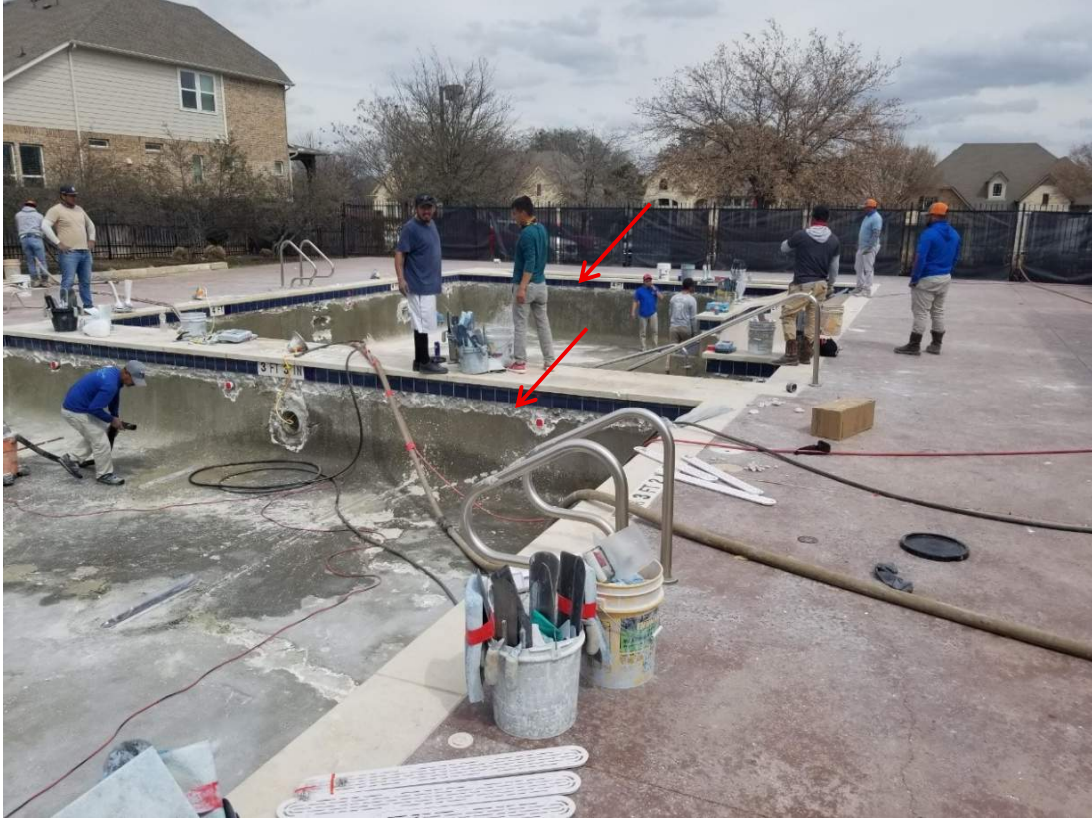
Photo No. 1 (2021)- Prior to plaster with bond coat applied. Rough chipped area under tile.
