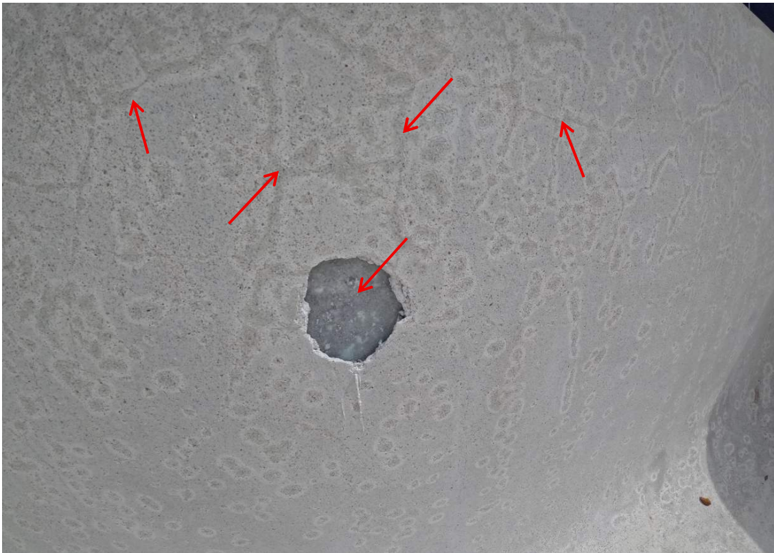
Photo No. 6 (2026) - This area had a thin bond coat and almost looks like epoxy on the wall. The spotting looks like it is pitting or spider cracks.
