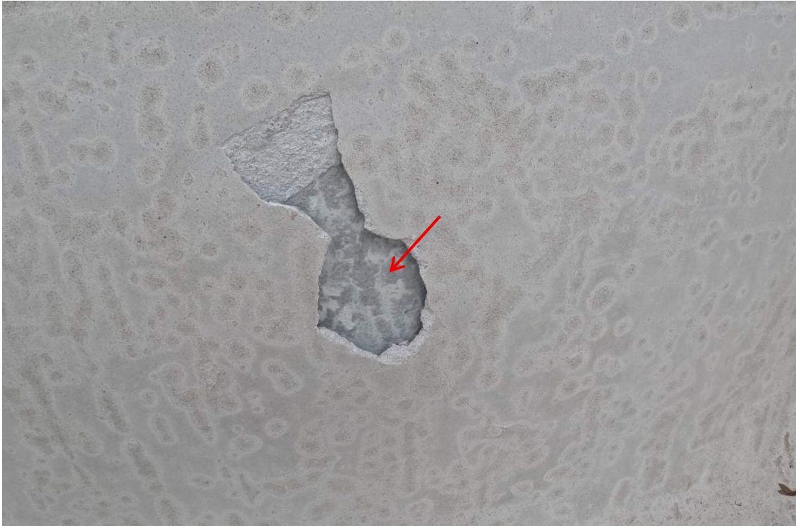
Photo No. 5 (2026) - Vanes of old plaster still in place under thin bond coat.
